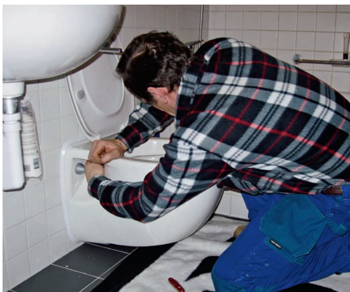
Connection to the future: A plumber installs a NoMix toilet in an apartment (Photo Timur Bürki)
