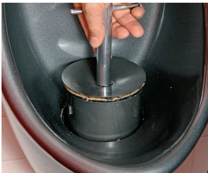
Essential maintenance: To prevent blockages, urinal components are exchanged according to manufacturer's recommendations (Photo Ruedi Keller)
